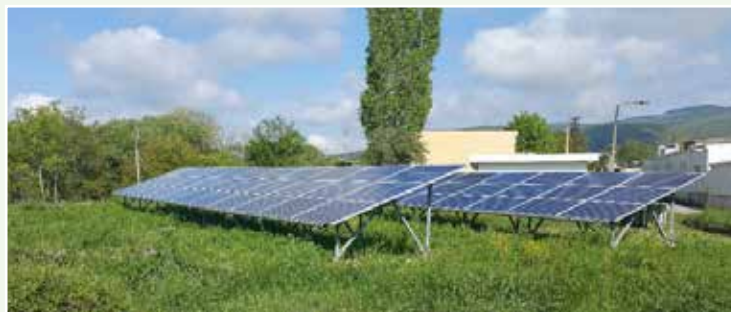
Solar panels at AQ Magnit, Bulgaria.
